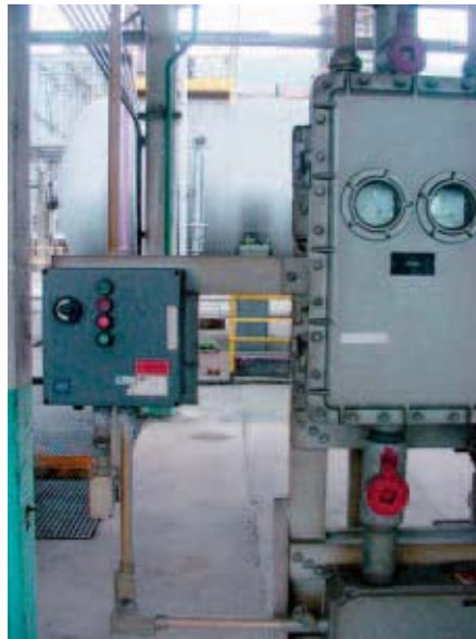
Figure 3: Non-metallic Ex ed control box of plastic material (left side) replacing Ex d old ones
