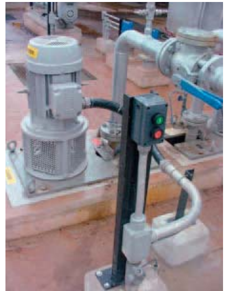
Figure 4: Control station made of glass-fibre reinforced material, type of protection Increased safety, 'e' and Flameproof enclosure, 'd' replacing the Ex d old ones, retaining the existing conduit installation
