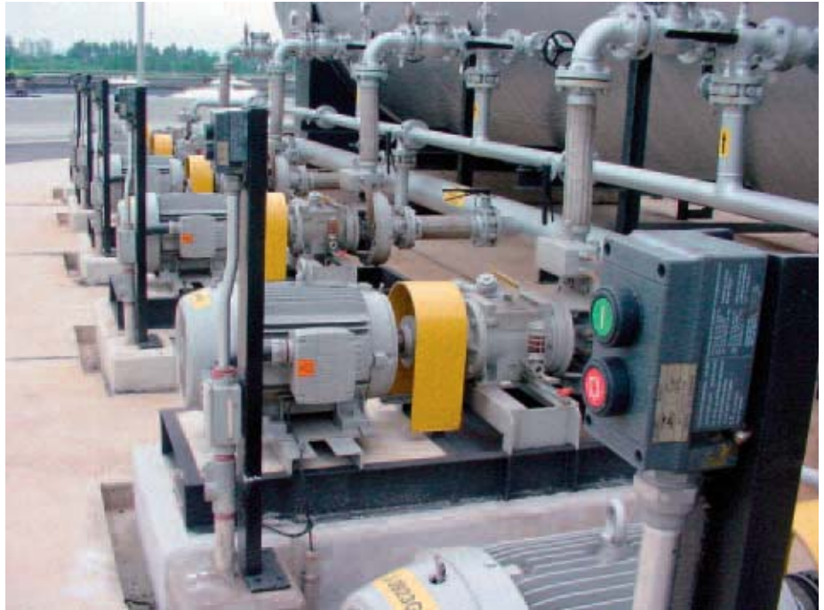
Figure 1: Control station in IEC technique for motor control
